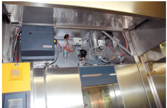
View of burner and electrical components above the oven.
