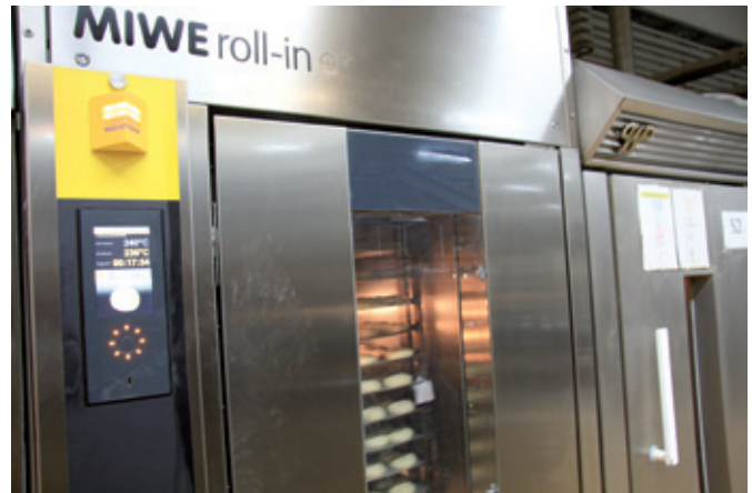
The MIWE roll-in oven’s control system is positioned separately, away from the hot baking chamber.
