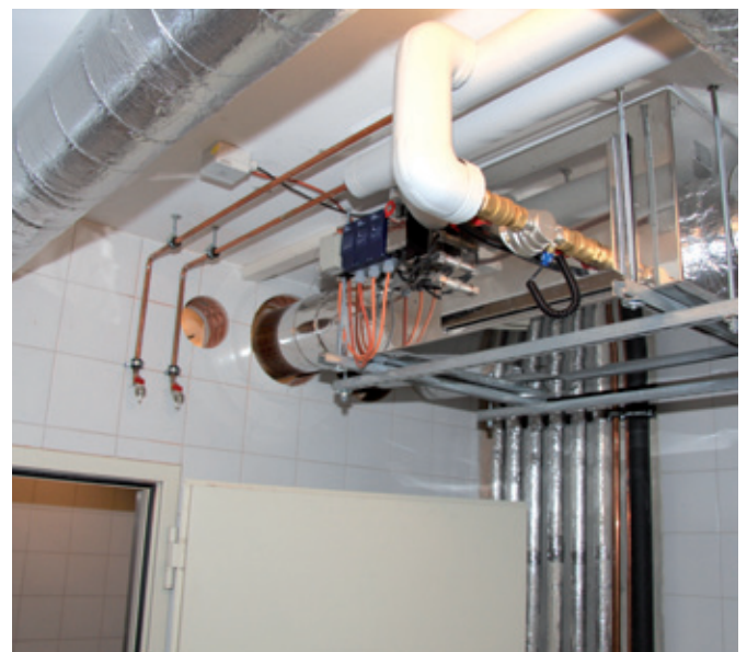
The waste gas pipes of the two rack ovens are directed into the MIWE eco:box in a side room.
